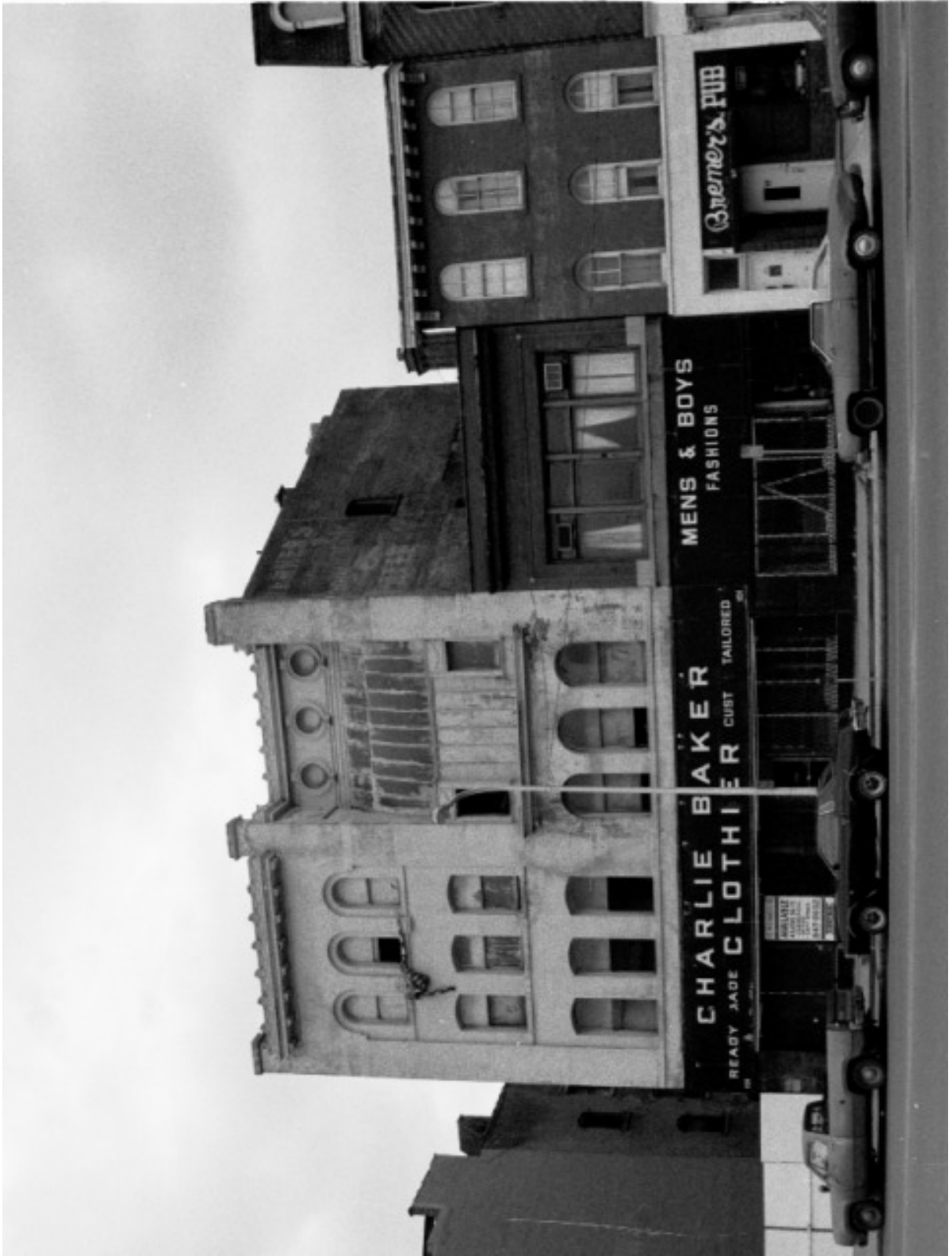
(7) The Werner Photography Building, ca. 1980 (Karl R. Josker, photographer) Note the deterioration of the waterfall window, the missing pinnacles and the modified storefront.
